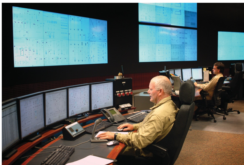
Figure 6.3 Picture of a typical centralized control room. (Photo courtesy of Worsley Alumina)
